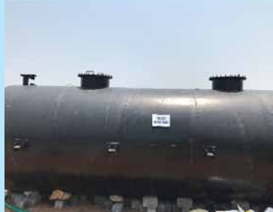
Treated Waste Water Tanks
