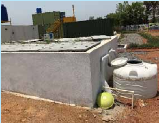
Waste Water Treatment
